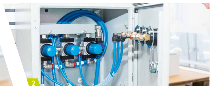
2 Control box - open
